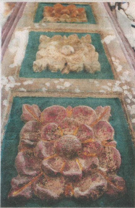
A closer look at a detail of the stone arch, which was painted upon. This has been painstakingly cleaned and the paint removed. Now it shows exposed stone like it would have originally sat along with door lintels. This has brought a sense of history back to the interiors.
